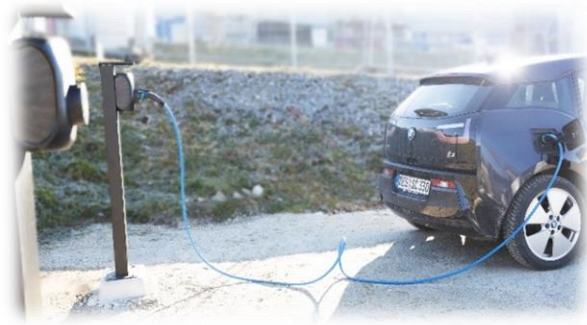
Electric vehicle charging points
